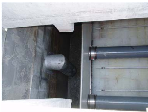
Figure 8 : Settled water channel
